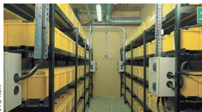
Battery technical plant application.
