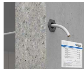
Wall feed-through in concrete fire-protection wall.
