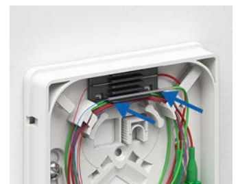
Perform splicing work and place the crimp splice protector in the holder.
