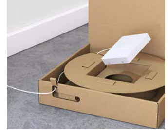
At the end, remove the optical termination outlet from the cardboard box and pull in the remaining cable.
