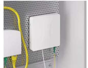
Example: Installation in the multimedia distributor.
