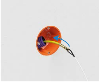
Connect the pull-in aid to the cable end and pull it into the empty duct.
