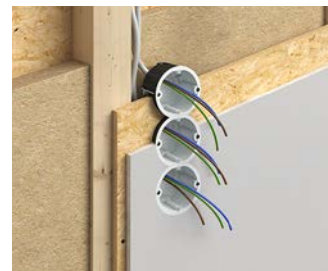
...in an F60-B wall, individual boxes up to a 3 box combination are possible.
