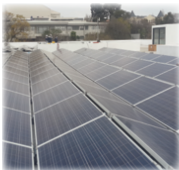
East-west mounting type- tin rooftop
